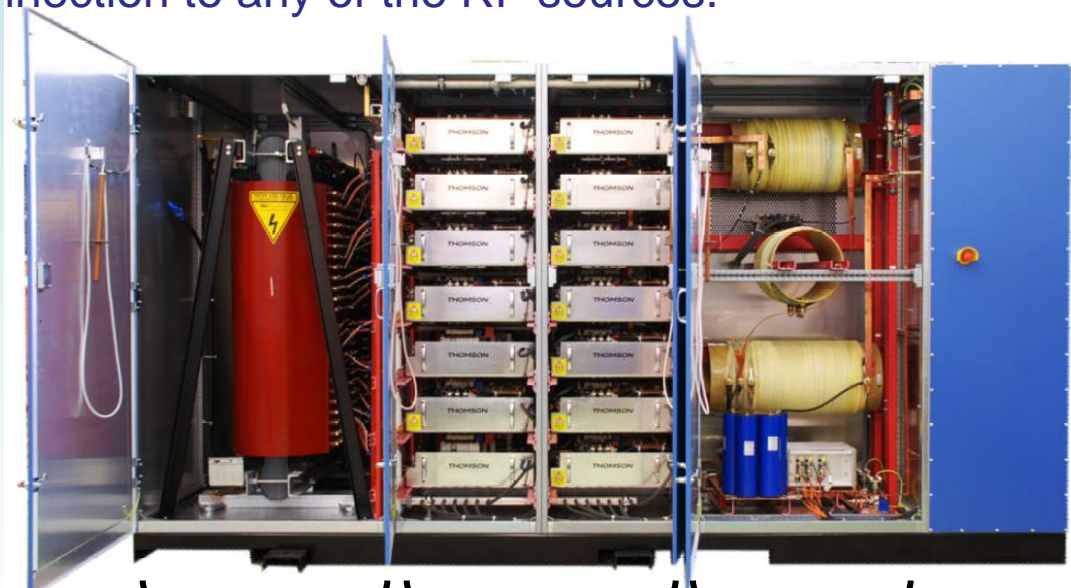
Transformer Modules Filter
