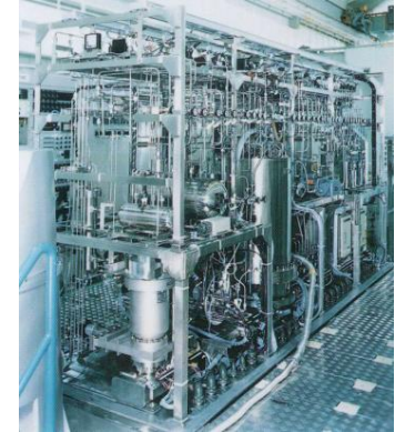
Fuel Clean-up System For TSTA
